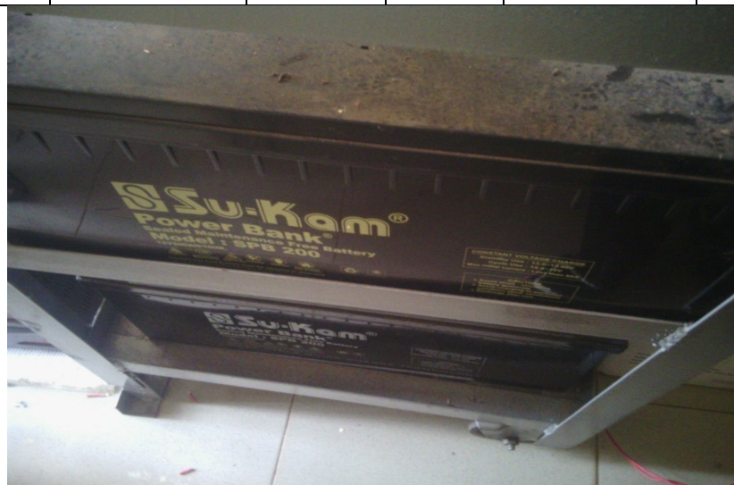
Figure 1: Su-kam Battery Setup
